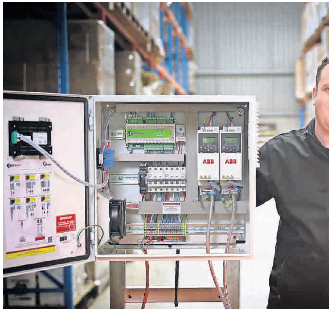
MATElec Australia's product manager Dale Jones with the HydroWHIZ control panel.
