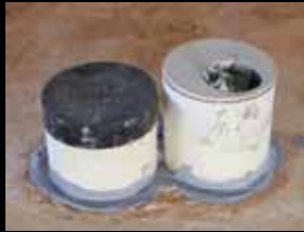
Penetration Void Filled with TERM-seal Sealant
